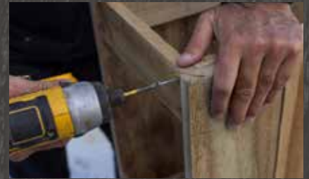
2: Create the frame for the hose reel cover by screwing the timber together to make a box, then add panel detailing.
