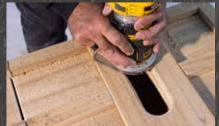
3: Create a hose slot and smooth the edges (so it doesn't puncture the hose). Drill a hole in the side of the cabinet wall for the hose connection.
